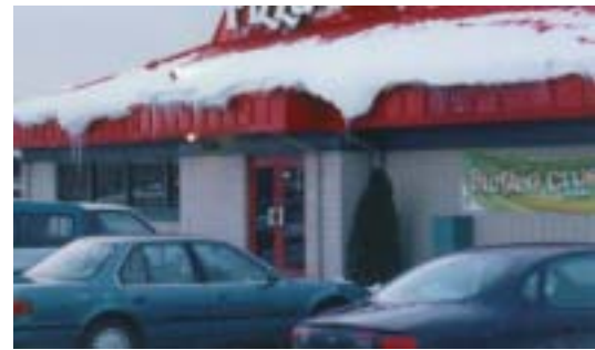
The snow above this entry door could release at any moment.
