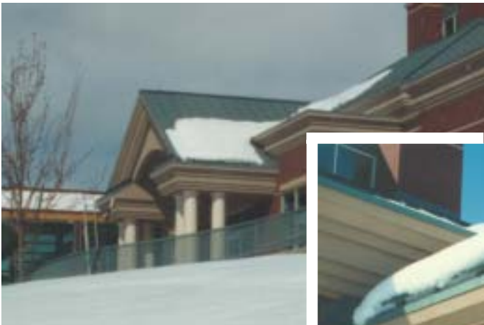
Snow sliding or falling from rooftops can be dangerous to vehicular and pedestrian traffic. Snow can easily weigh 15 pounds per cubic foot or more. A 20-foot by 40-foot roof with an 18-inch deep blanket of snow suddenly avalanching can send as much as ten tons of snow crashing onto whatever is beneath it. It can tear off eave gutters and damage other building elements, as well.
