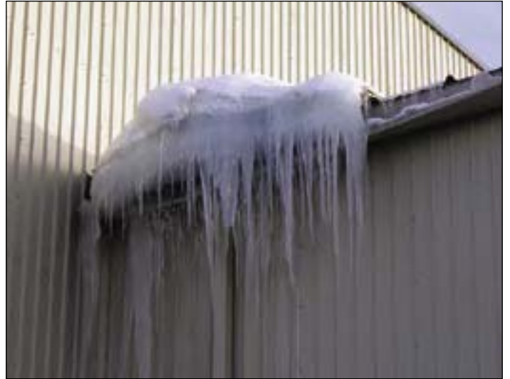
Gutter left unprotected cannot resist sliding ice and snow.
