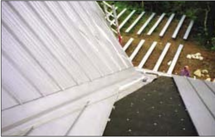
The back side of the church has no snow retention. The result is severe roof damage due to sliding ice and snow.
