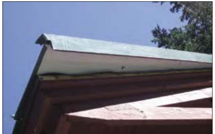
...forcing the roof approximately 6" out of plane laterally.
