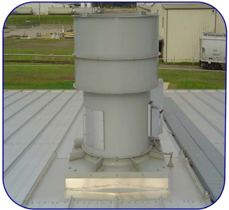
Above: Exhaust Fan with correctly installed curb.
